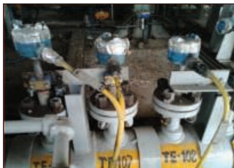
FIGURE 9. A view of the final configuration of the piping shows additional pipe supports
