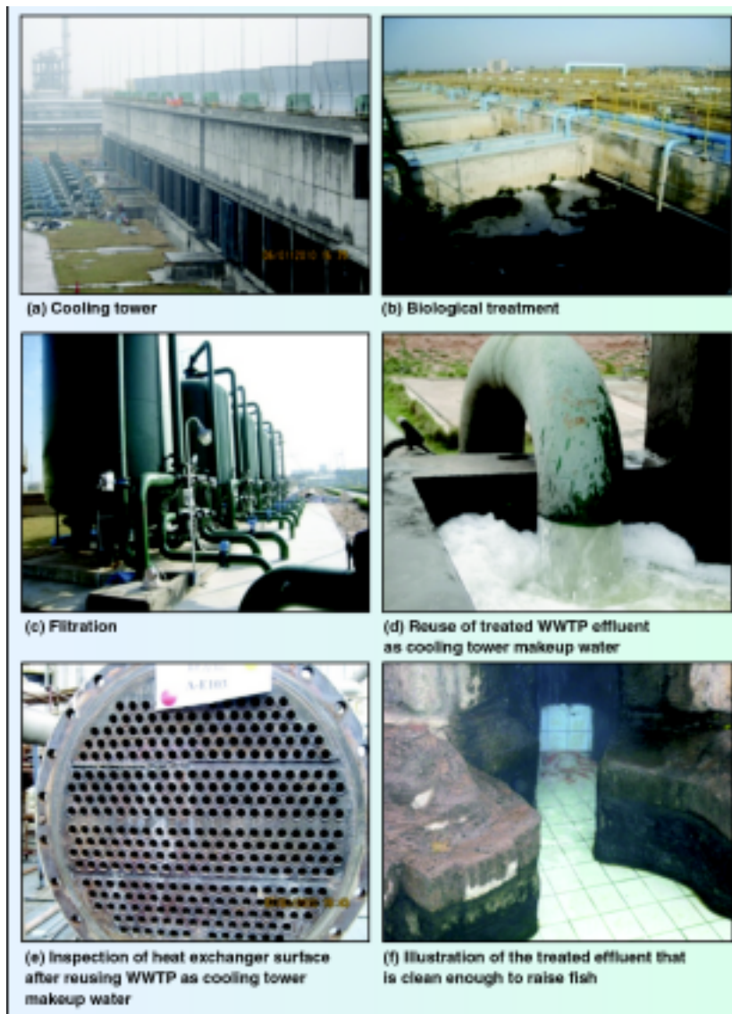
FIGURE 7. Photos from a large ethylene plant illustrate how treated WWTP effluent can be reused as cooling-tower makeup water
